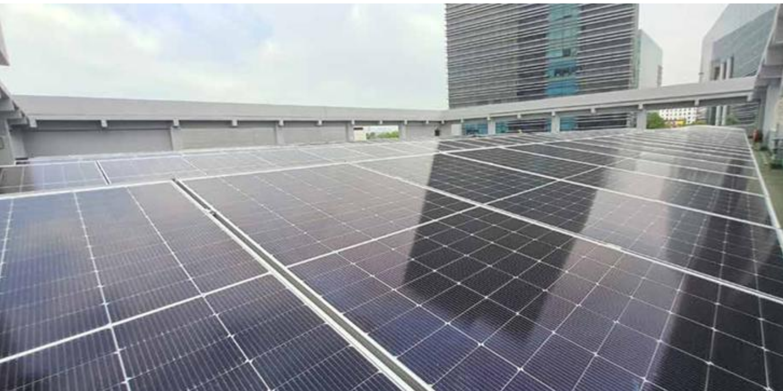
Solar panels at mTower, Singapore
