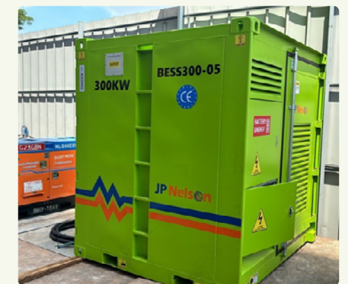
BESS at Mapletree Joo Koon Logistics Hub, Singapore.
