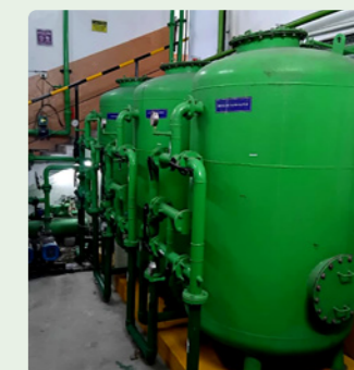
On-site Water Treatment Plant at Global Technology Park, Bengaluru.
