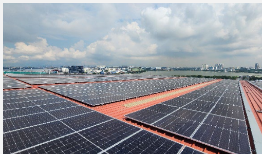
Rooftop solar panels at 4 Pandan Avenue
